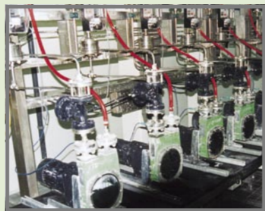
■ Water treatment - Lime dosing
