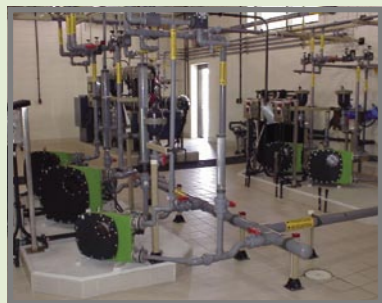
■ Water treatment - Dosing hypochlorite
