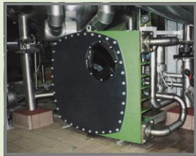
■ Brewing - Pumping shear sensitive yeast
